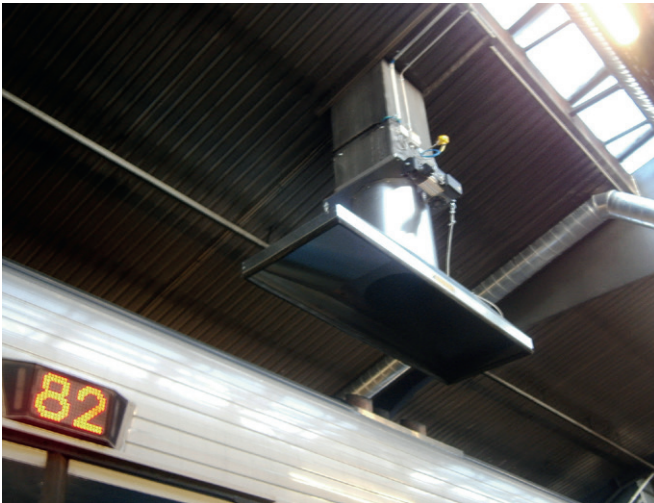
Extraction Hood for train
