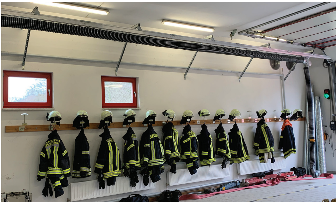
MRSP installed in a fire station
